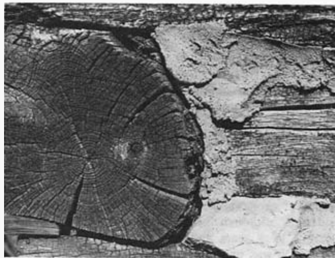
Figure 29 —Deep checking on an old log structure retains moisture and encourages decay.
