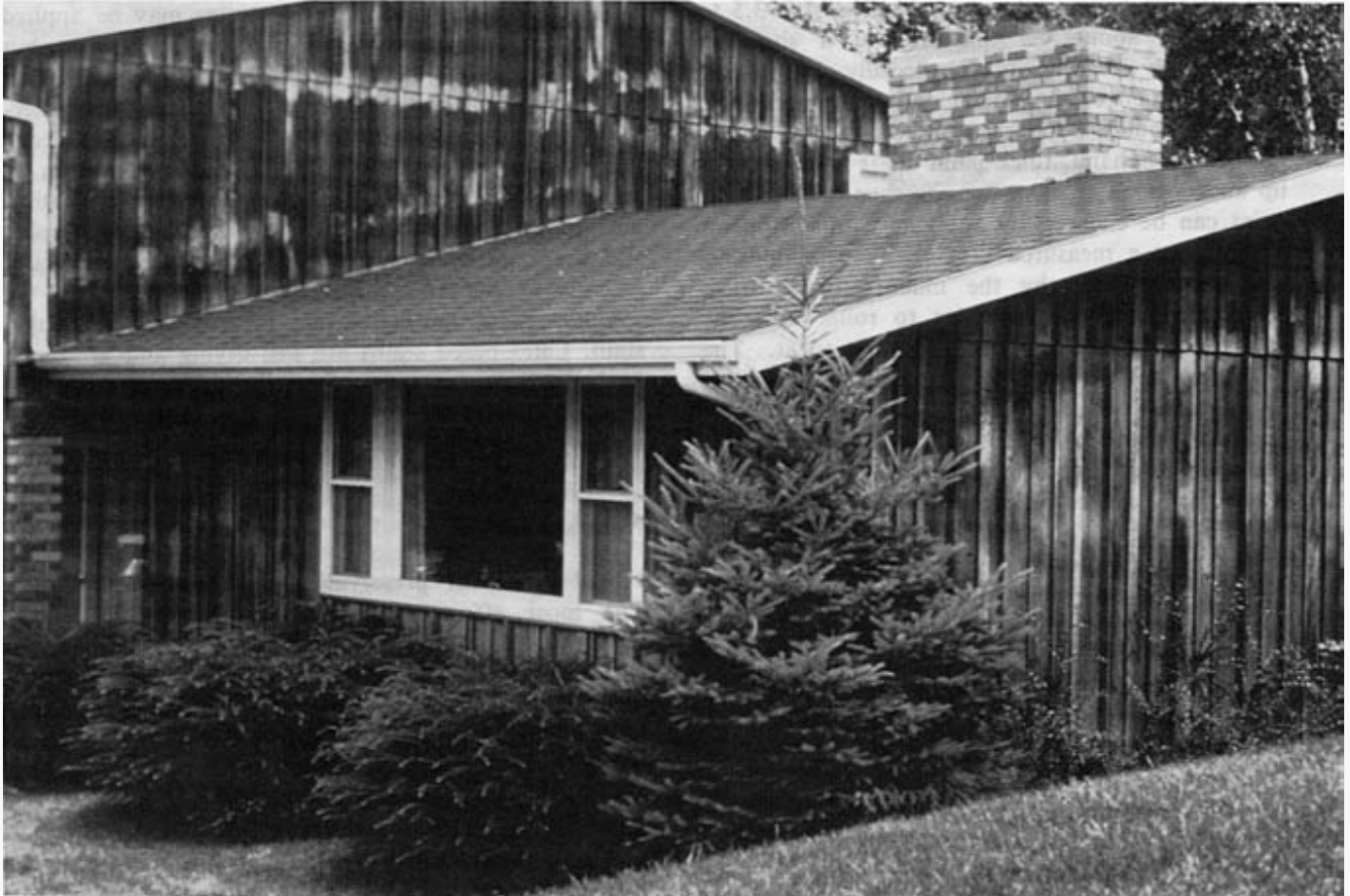
Figure 26 —Lap marks formed by improper application of a semitransparent penetrating stain.
