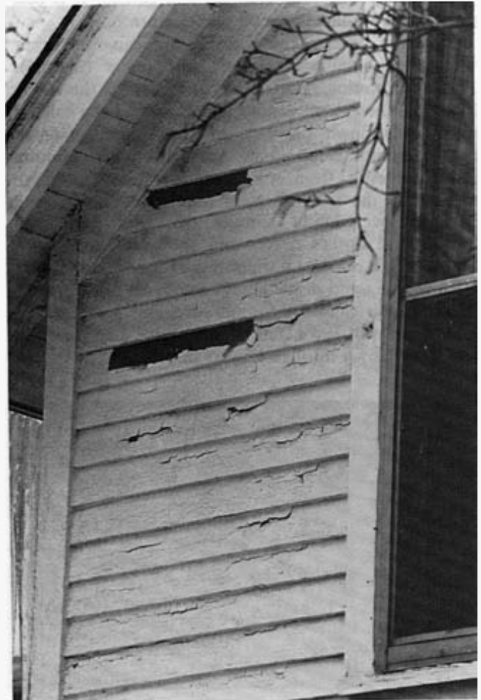
Figure 35 —Paint peeling from wood can result when excessive moisture moves through the house wall. Some cross-grain cracking is also evident on this older house.
