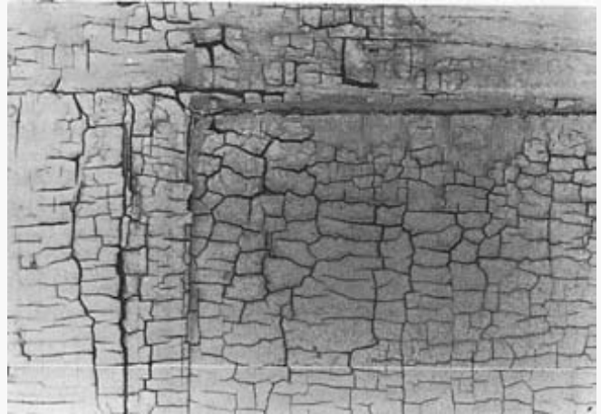
Figure 33 —Cross-grain cracking results from an excessive buildup of paint.
