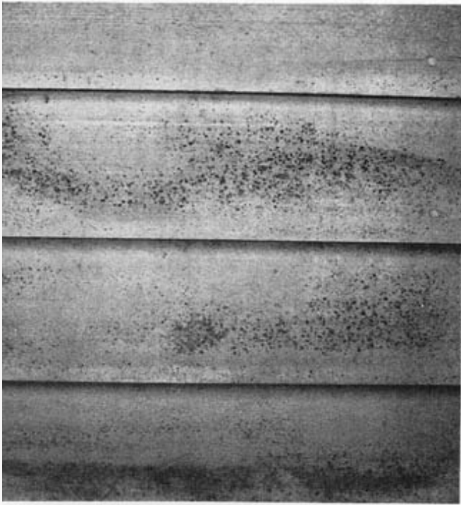
Figure 31 —Mildew on paint is most common in warm humid climates as well as in shaded or protected areas.
