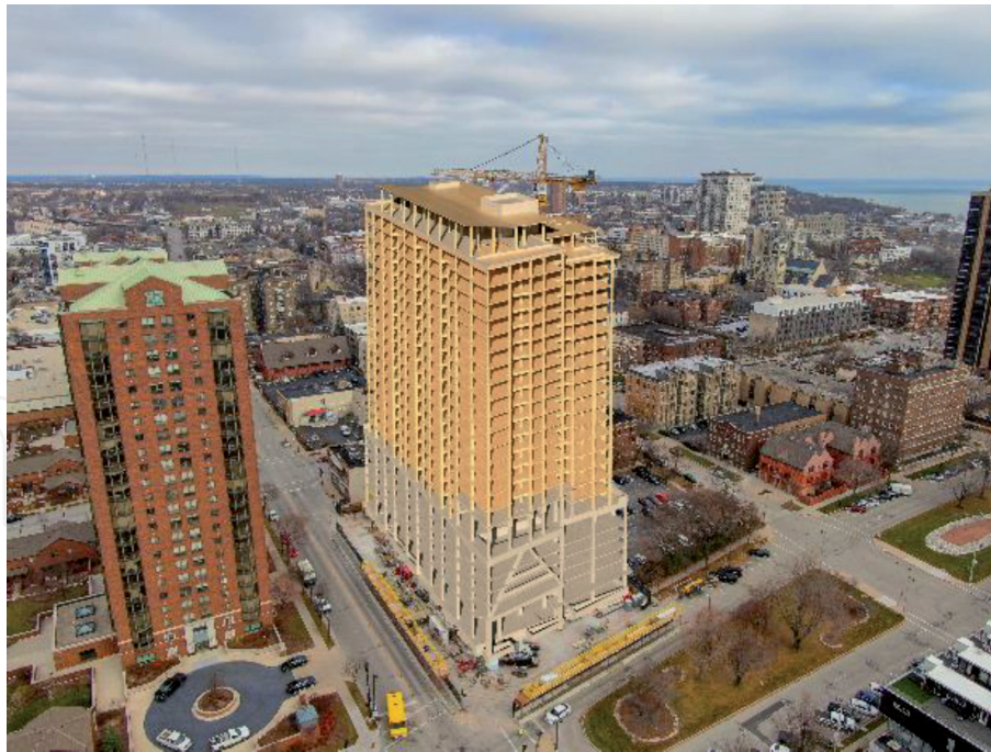
Figure 2. 25-story Ascent building built with mass timber products in Milwaukee Wisconsin US (Credit: Thornton Tomasetti and Korb & associates).
