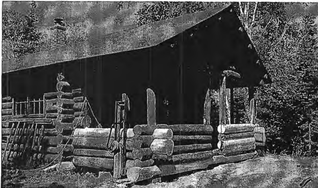
Figure 8 - Replacement of decayed logs sections on the front and left side of the Bearskin guard cabin. The new logs are light colored and clearly match the decayed sections as identified in figure 1.
