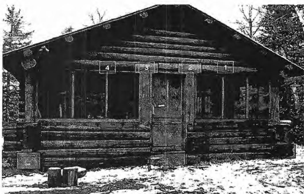
Figure 3 - Bearskin cabin front showing decayed sections as identified through visual inspection, stress wave timing and resistance drilling. Dark shading reflects areas of severe decay and light shading areas of moderate decay.
