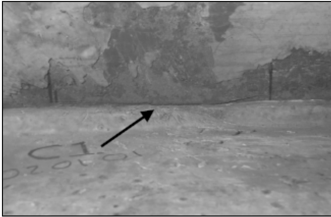
Figure 5 Longitudinal crack at weld toe
