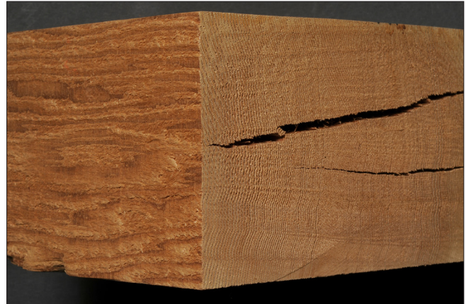
Figure 13–11. Red cedar timber end shows honeycomb (top). Surface of the timber shows no honeycomb (bottom).
