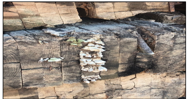
Figure 5—Fungal fruiting bodies on the end-grain of a glue-laminated mat timber. These fruiting bodies indicate advanced decay. The strength of this timber is thus significantly reduced and warrants further inspection and evaluation. Photo is property of Mississippi State University.
